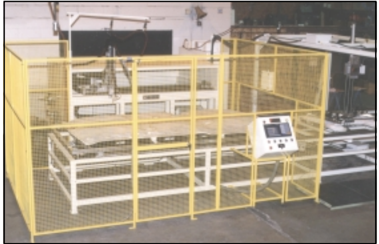
The headliner in the dispense position surrounded by e-lock guarding.
